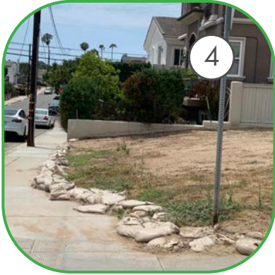
Most critical drainage issue. To be addressed with Sustainable Urban Drainage System
